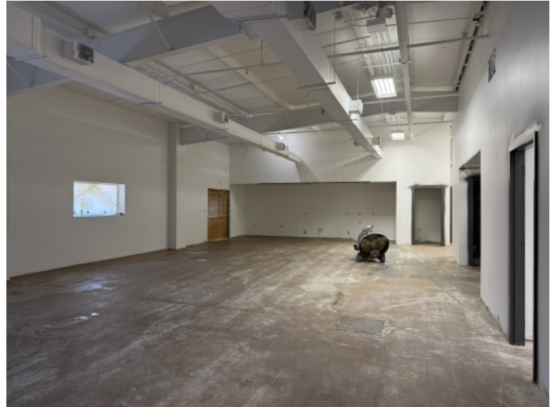
TRANSPORTATION BUS DRIVER BREAKROOM AREA
